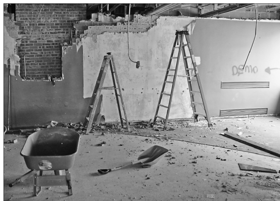
Tulsa-based Flinto has completed demolition on two floors of downtown Tulsa's 135,000-square-foot Central Library, with two more underway, said Gary Shaffer, CEO of the 24-branch Tulsa City-County Public Library system. During a Friday tour of the construction site, Shaffer said he foresaw a spring 2016 reopening for what had been the organization's busiest facility, with more than 400,000 visitors each year. The 48-year-old structure will retain the overhanging canopy and dramatic support columns designed by original architects Charles W. Ward and Joseph Koberling, while modernizing its environmental systems and infrastructure. COURTESY PHOTO BY JOHN FANCHER
